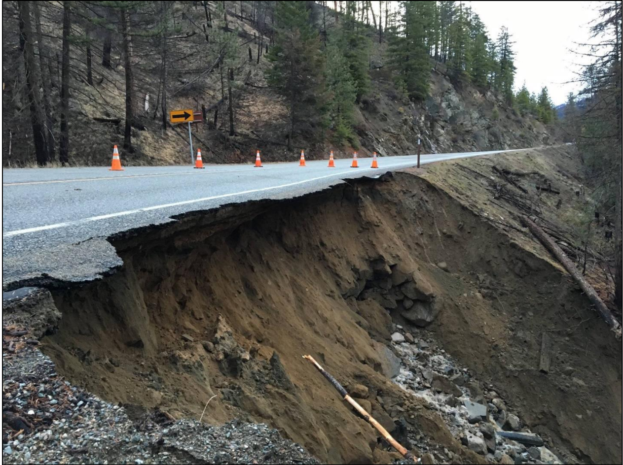
Figure 30) Damage to SR 20 in Okanogan County, WA caused by a landslide that took place on April 8, 2017. “Okanogan County Emergency Management reports a slide that has closed State Route 20 at mile marker 221.7. In a Facebook post they tell us the roadway is very unstable and the damage is 70 feet wide. To detour around the slide, use State Route 153.” Photos were taken by Okanogan County Emergency Management and were originally posted on the Fox Q13 website on April 8, 2017. The original story and photos can be accessed at the following URL: https://q13fox.com/2017/04/08/sr-20-closed-near-okanogan/
